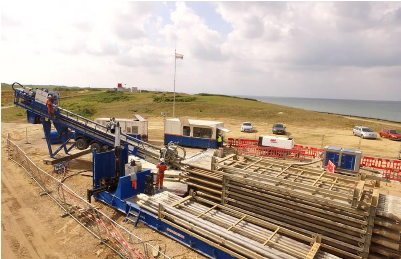
Plate 5-12: Example of an onshore landfall compound (Dudgeon OWF) with drilling rig (left of shot) in operation (Source: Equinor)
